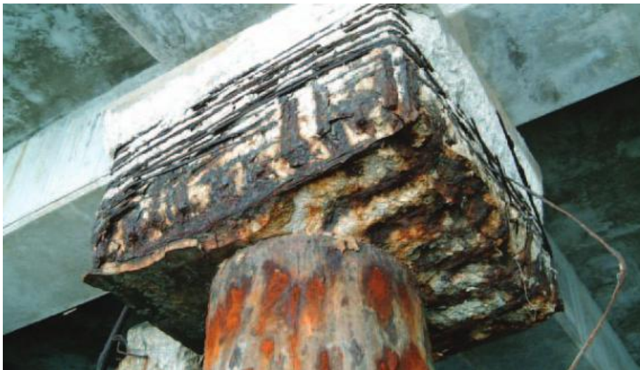
Fig. 1. Destruction of concrete and corrosion of reinforcement
